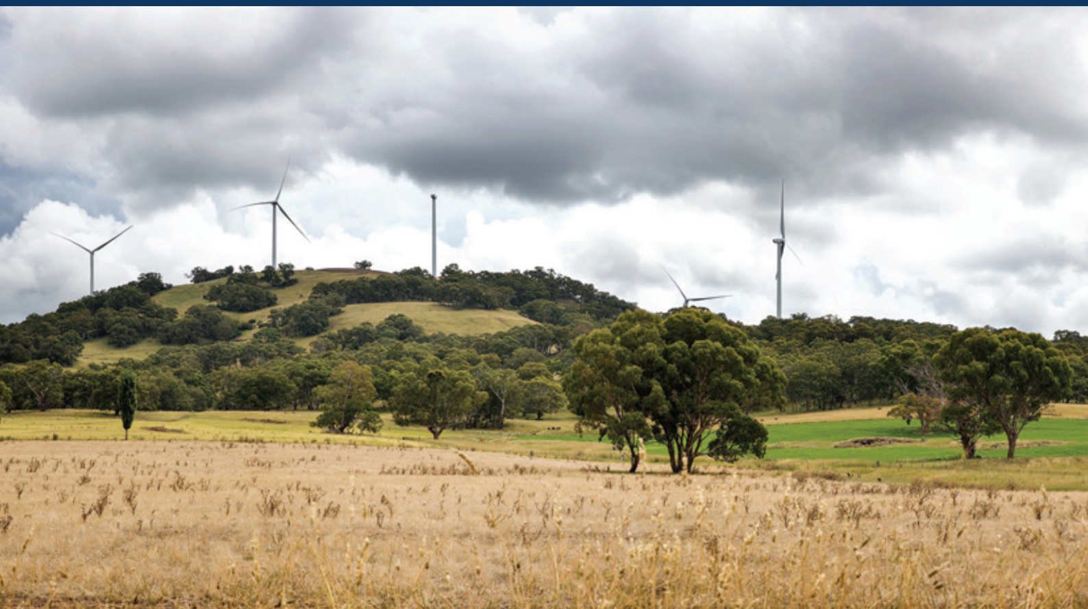
View of White Rock Wind Farm turbines in various stages of installation from Jenkins Road
